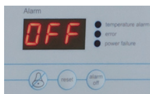
Display showing alarms turned off
